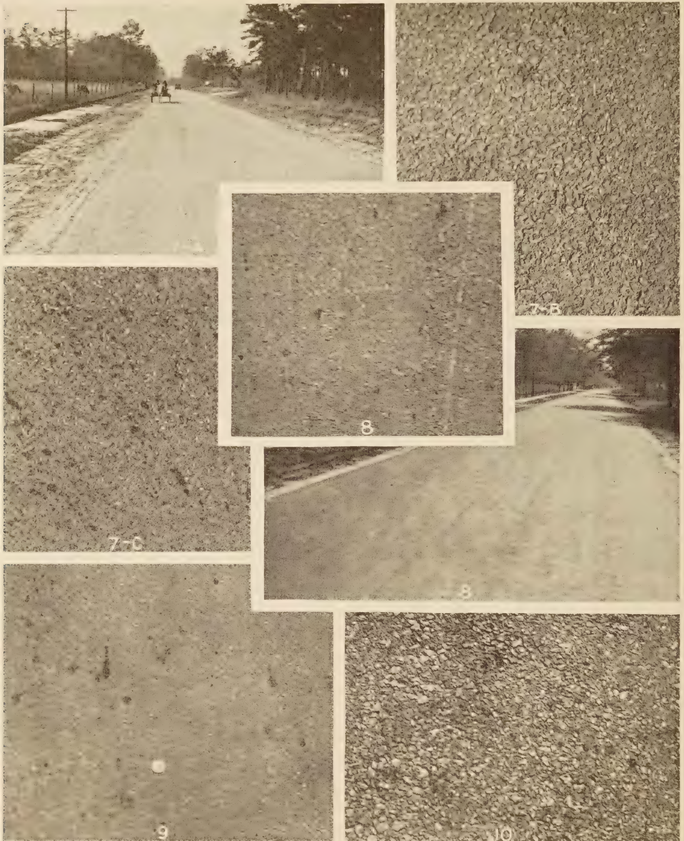
FIGURE 8.—TYPICAL EXAMPLES OF SURFACE CONDITION DURING THE SPRING OF 1931. THE NUMBERS OF THE EXPERIMENTAL SECTIONS ARE GIVEN ON THE PHOTOGRAPHS
